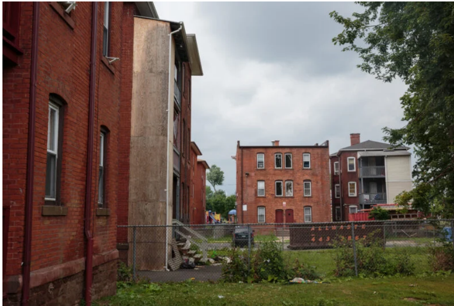
Before HUD ended its funding contract, the Clay Arsenal Renaissance Apartments in Hartford had passed its HUD inspections despite tenant complaints about conditions. (Sarah Blesener, special to ProPublica)
